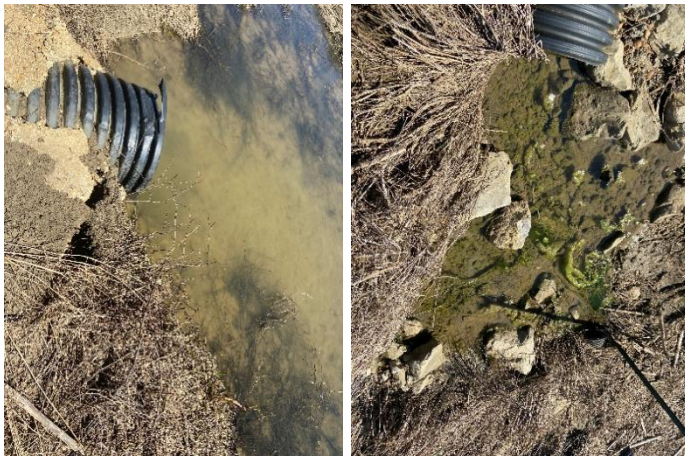
Fig. 3. Outlet of existing subsurface drainage pipes on Good Farm in March, 2023
